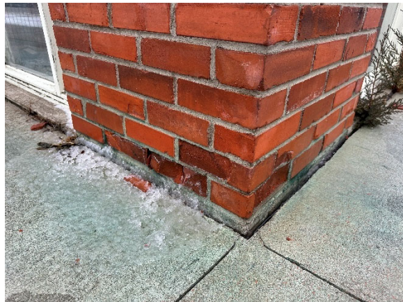
Brick Deterioration at Grade
