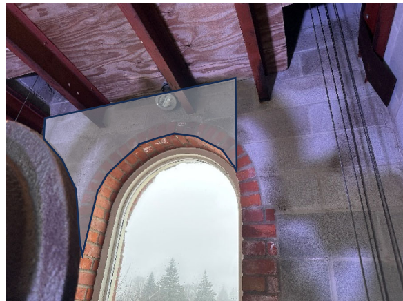
Wet and Spalling Interior Block
