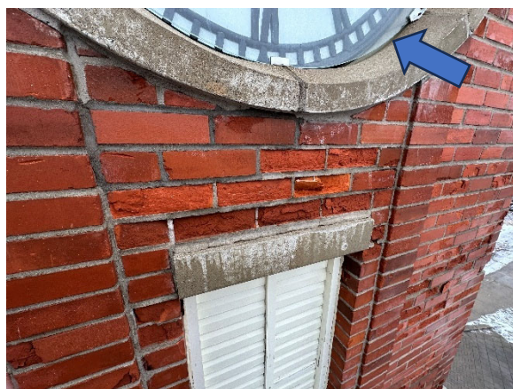
Brick Deterioration Vented space between storm glass and surround
