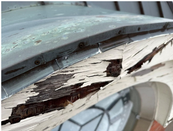
Wood Fascia Deterioration
