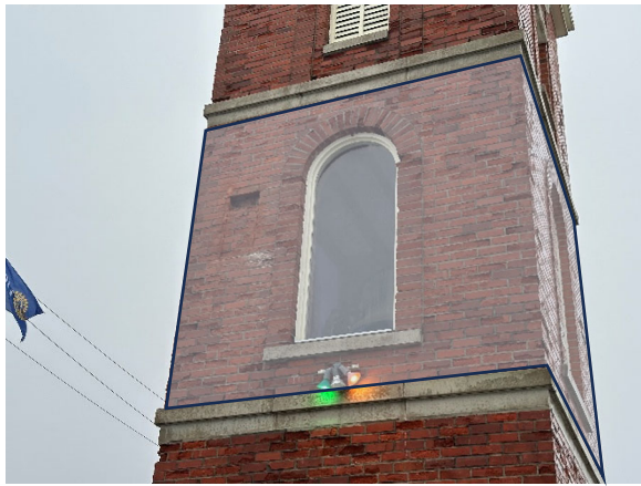
Partial West Elevation Deteriorated brick units
