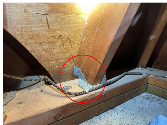
Improper Tie Down Anchors Grounding cable
