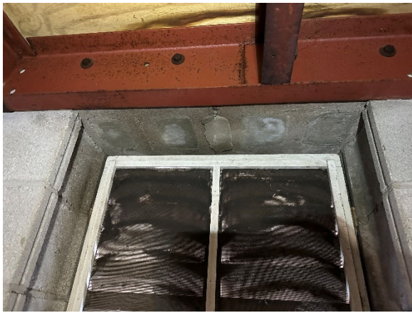
Wet Interior Block at Louvre Opening Block is saturated with moisture
