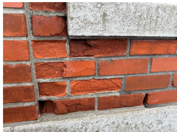
Brick Spalling @ Window Sill
