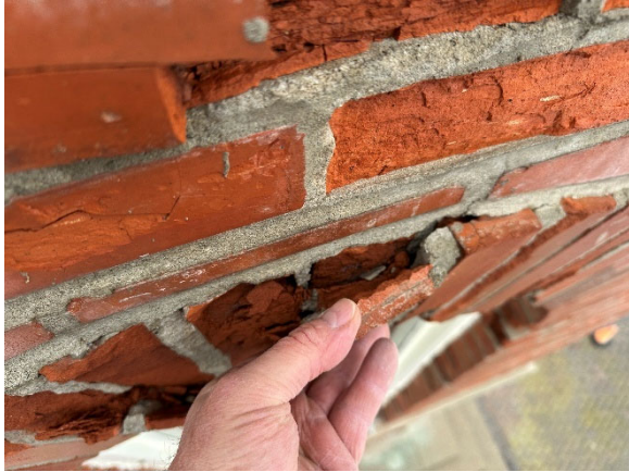
Brick Spalling @ Window Arch
