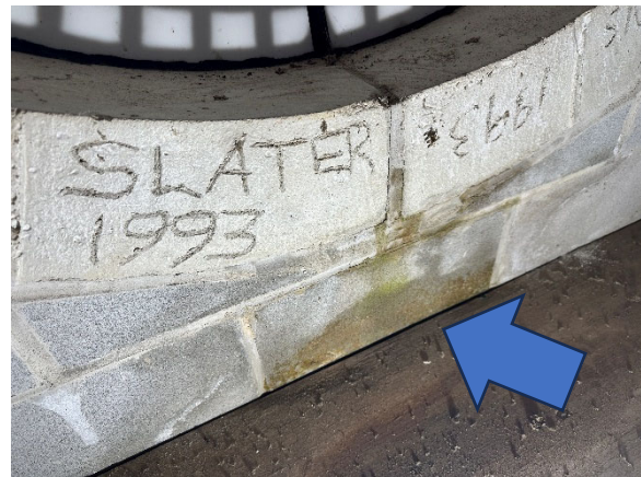
Interior Sill @ Clock – Water Ingress
