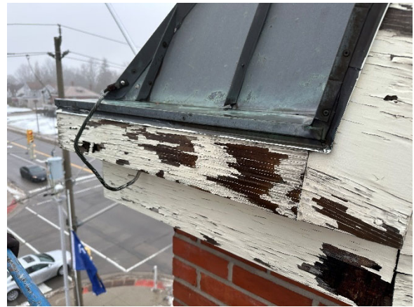
Wood Fascia and Trims Deterioration
