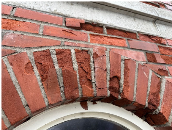
Window Header Brick Deterioration
