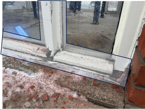
Wood Screen at Grade Deterioration
