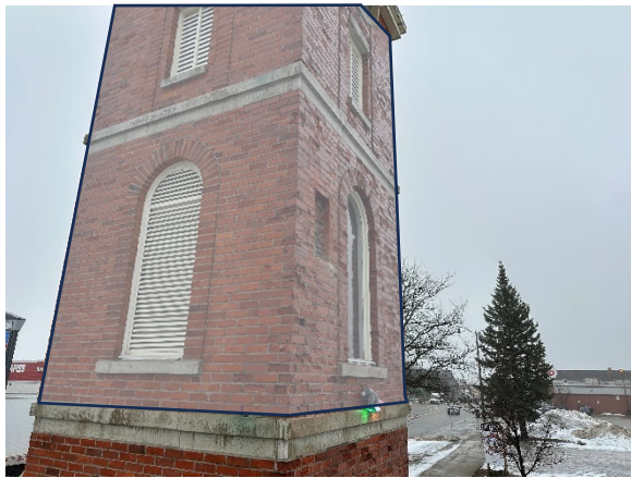
North (left) West (right) Elevation Masonry Deterioration
