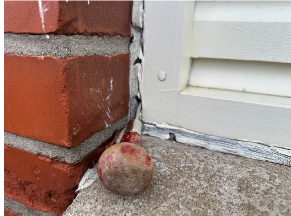
Deteriorated Sealant @ Louvre
