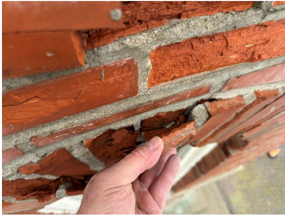
Brick Spalling @ Window Arch
