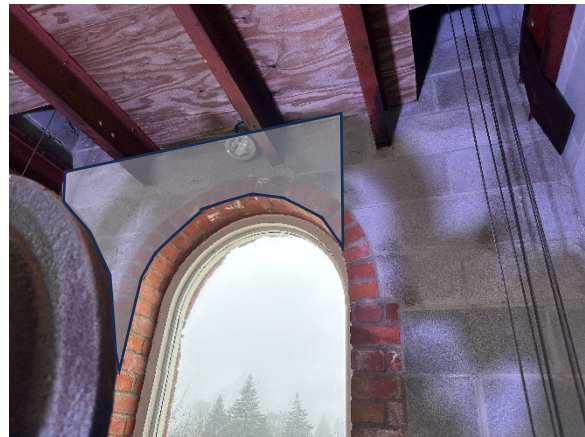
Wet and Spalling Interior Block
