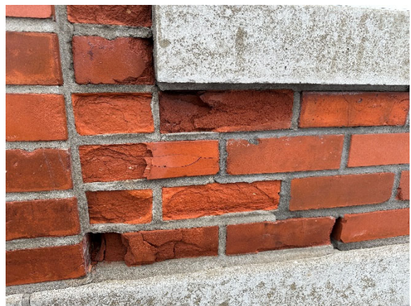
Brick Spalling @ Window Sill
