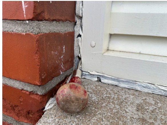
Deteriorated Sealant @ Louvre
