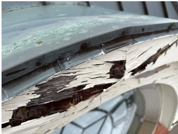
Wood Fascia Deterioration
